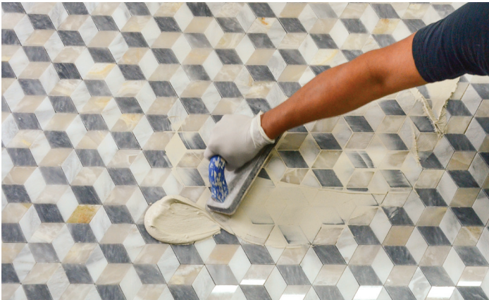
Step 8 Apply grout with a rubber grout float, forcing grout into joints until full. Remove excess grout with edge of float.
