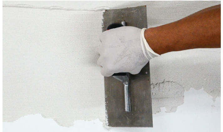
Step 2 To establish the proper depth of the setting bed, use a 3/16" x 1/4" v-notch trowel to apply additional thinset and comb full notches in one direction.
