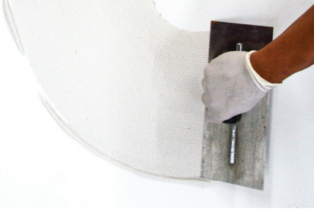
Step 1 To initiate the bond coat, use the flat side of a trowel and firmly apply thinset to the substrate.
